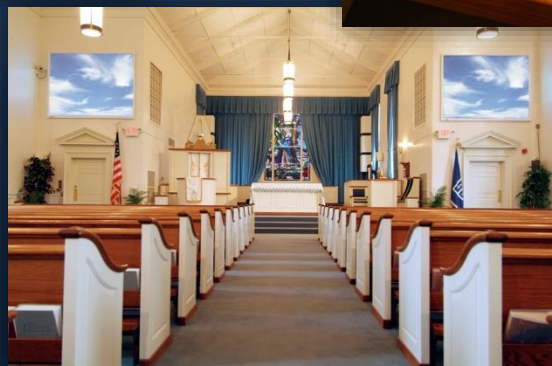
Dept. of the Army – Fort Belvoir Chapel AV System Install and Crestron Control Module
